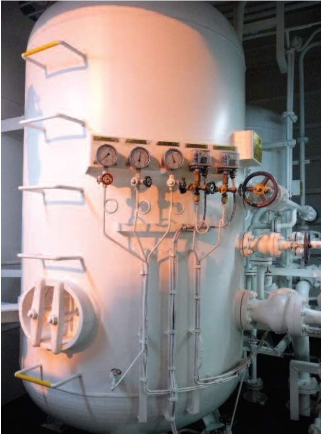
Depleted air bottles: Excessive numbers of engine starts/stops during manoeuvring will deplete pressure in the main engine start bottles which can result in loss of control of the vessel at critical times, such as when docking, due to the engine failing to start.
