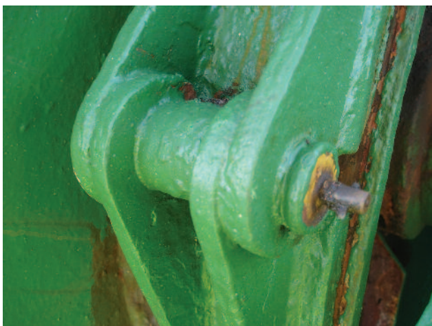
Ineffective grease point
