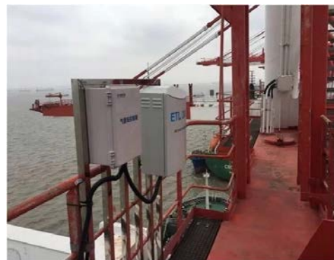
(Detecting device installed on shore crane)
