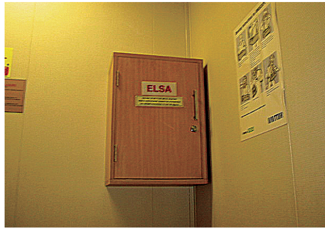
Good position at accommodation stairwell, but wrongly marked.
