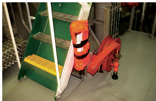
Good position in engine room
