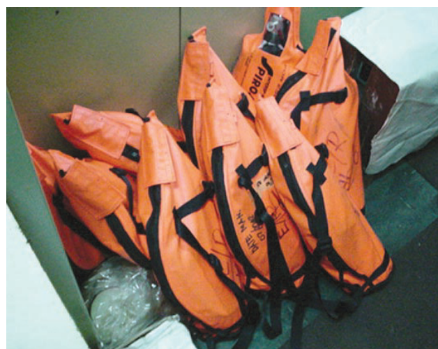
Badly positioned EEBDs, all together behind engine room switchboard
