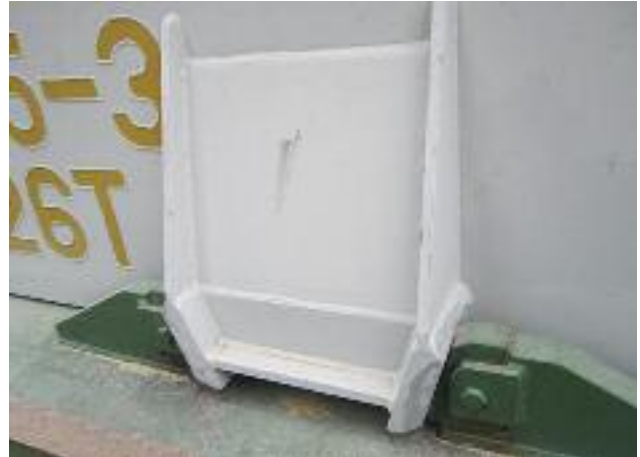
Properly maintained and adjusted locator
