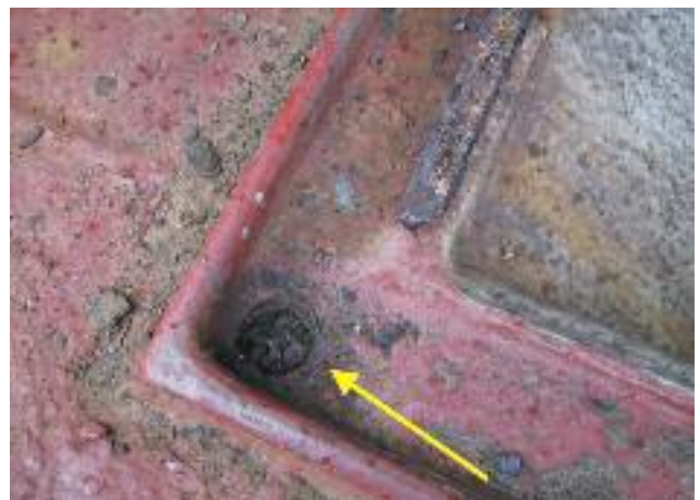
Presence of rust and debris will eventually lead to the clogging of the drain hole/drain pipe
