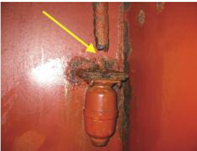
Corrosion wasted drainpipe
