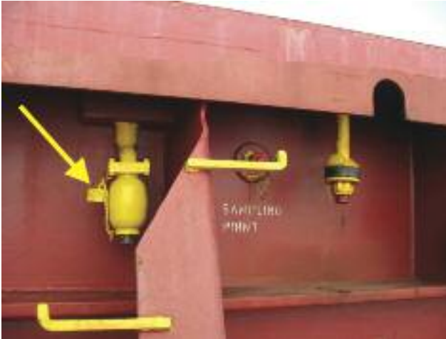
Drain valve (yellow) with threaded fire cap firmly connected by a lanyard
