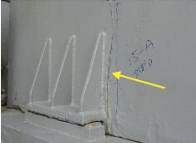
Improper repairs to bearing pad and a crack developing in the hatch panel side plating due to advanced bearing pad wear
