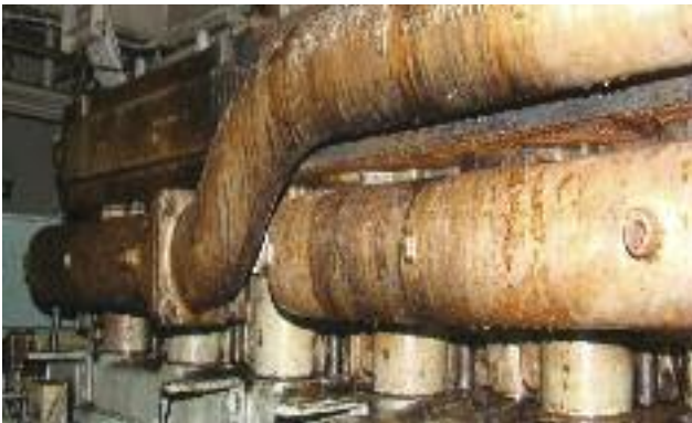
Exhausts completely uninsulated
