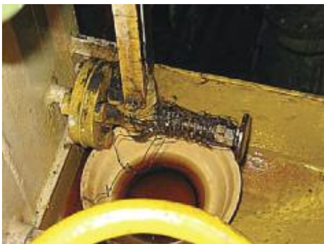
Self-closing gauge glass valve gagged with wire
