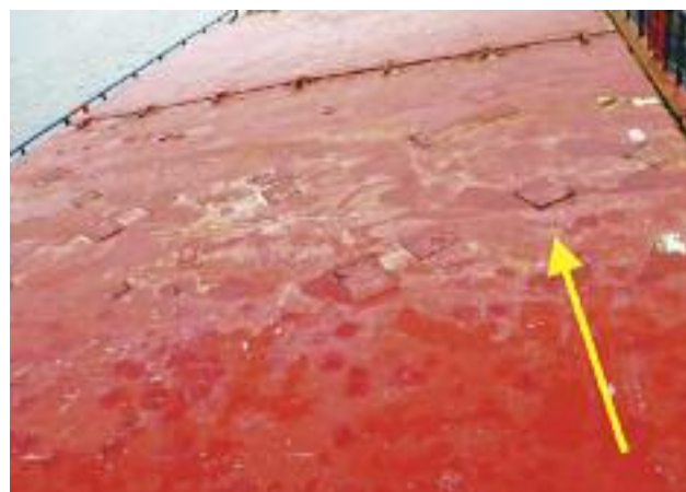
Multiple doubler plates on the hatch top plating
