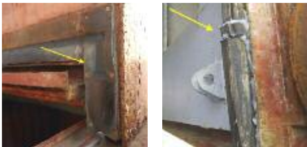
Backing strips (here nailed into the original packing rubber) and short insert repairs are frequently seen as evidence of improper repairs
