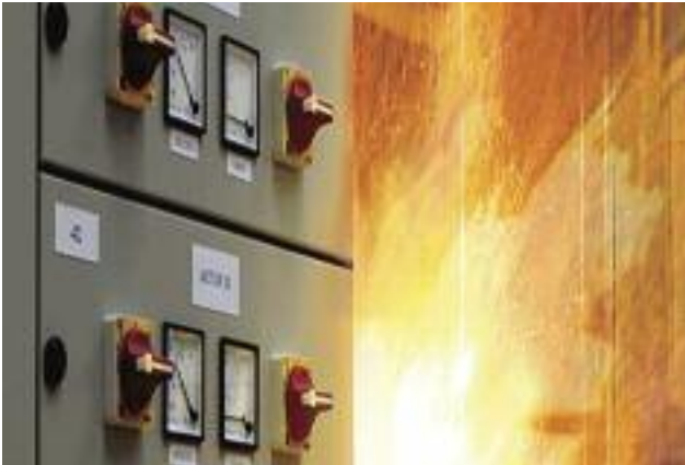
Arc flash incident
