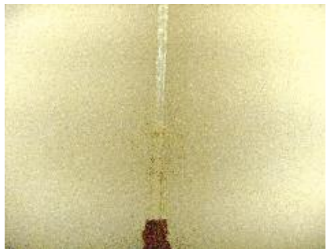
Cracking in paint over weld
