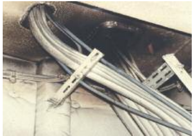
Cables entering a distribution board through fire stopped openings in the casing
