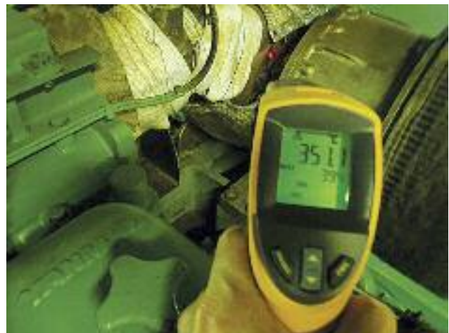
"Hot spot" due to missing insulation
