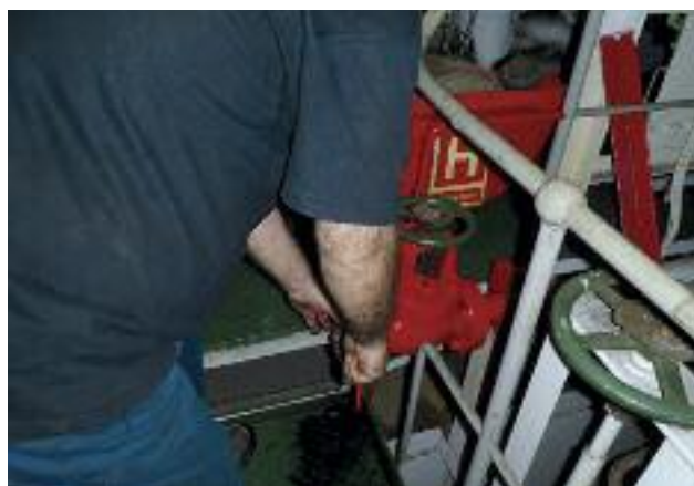
Hydrant cap difficult to remove, and valve leaking
