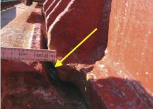
Excessive clearance in way of stoppers
