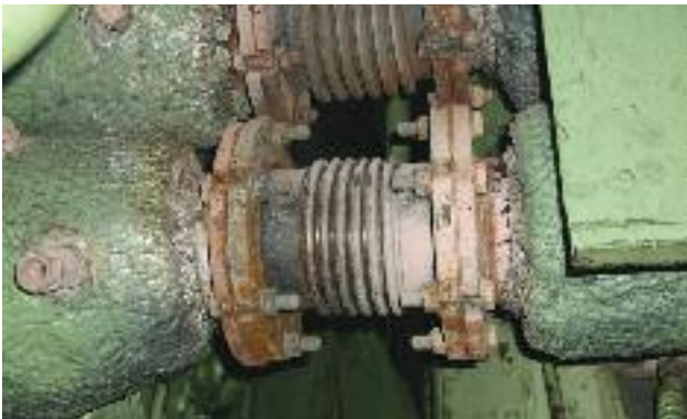
Exhaust bellows exposed
