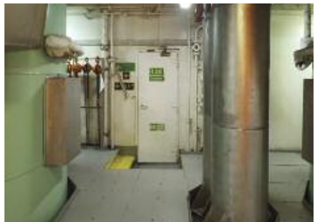
Poorly marked escape route and door
