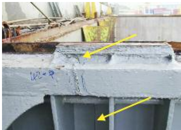
Crack progressing from the landing pad into the coaming
