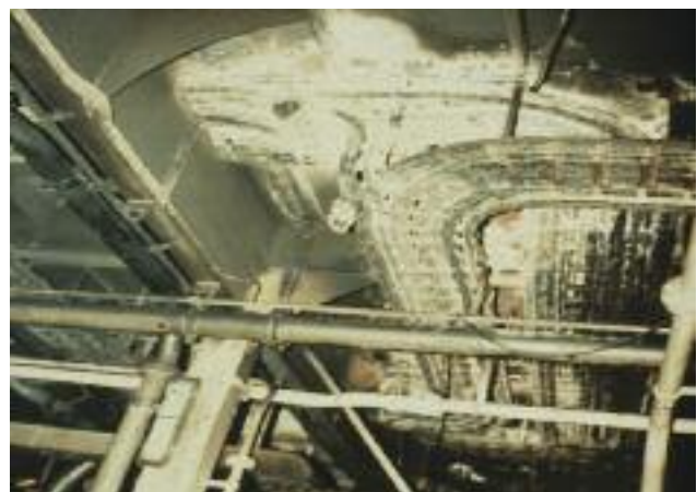
Damage caused by the spread of fire along cable trays after being exposed to a fire at a lower level of the engine room.
