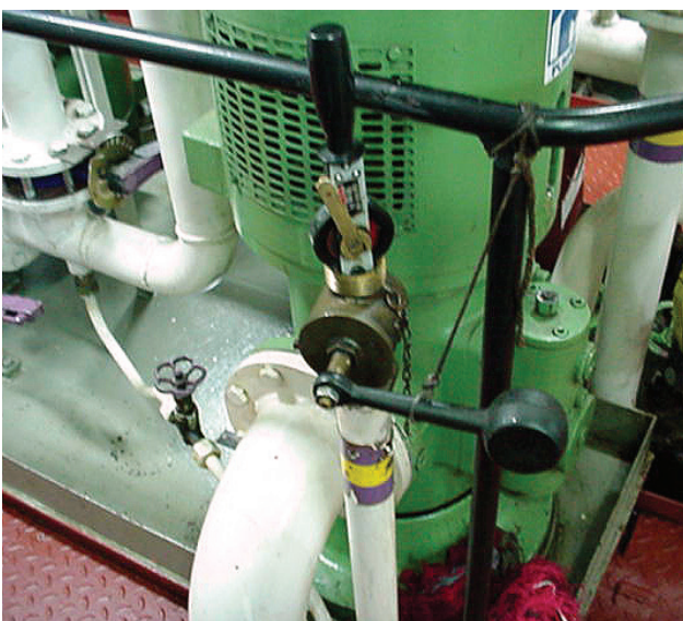
Tape left in lashed open sounding pipe
