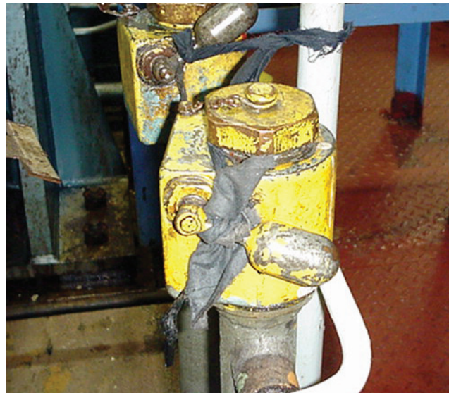
Sounding pipe lashed in an open position
