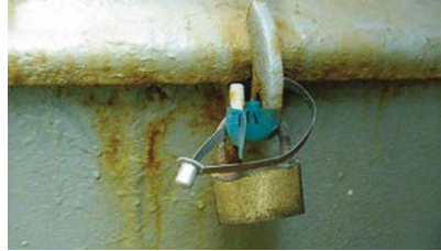
Figure 1.26: Security seal in place.
