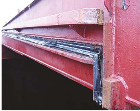
Figure 1.13: Poor practice: use of hatch tape to build up a cross joint is discouraged.
