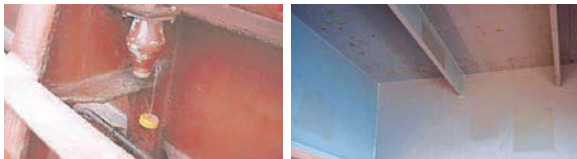
Figure 1.8: Hatch drain with cap attached by small chain.
