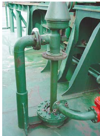
Figure 1.2: Hold cleaning equipment in the stowed position above the deck. Note the flange on the deck wash line.
