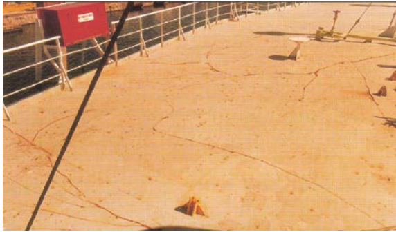
Figure 24.5: Brittle fracture of a ship's deck resulting from an LNG spill.
