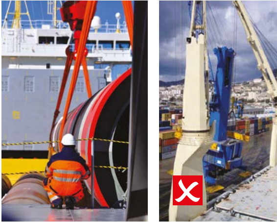
Figure 45.27: Unsafe lifting equipment.
