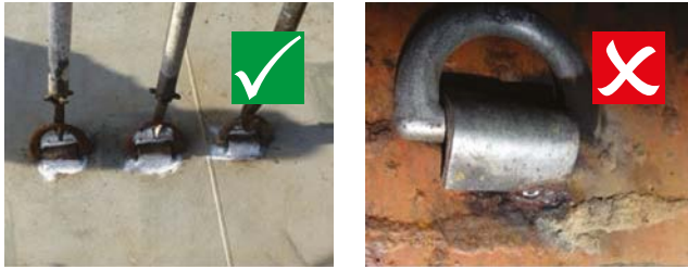
Figure 45.23: Examples of D-rings properly welded to the deck (left) and poorly welded onto a bulkhead (right).
