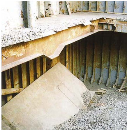
Figure 51.4: A collapsed tween deck.
