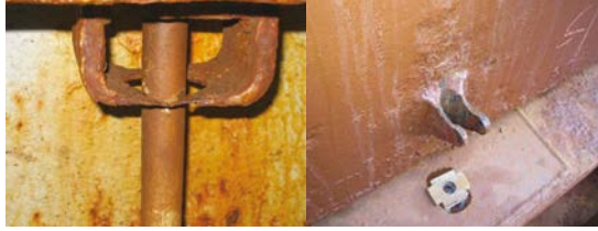
Figure 55.17: Corrosion of quick acting cleat crutch (left), thinned down snugs (right).
