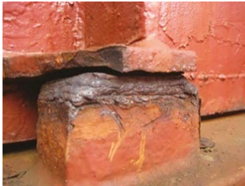
Figure 54.12: Improper repair to a bearing pad.
