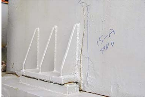
Figure 55.11: A crack developing in the side plating due to advanced bearing pad wear.
