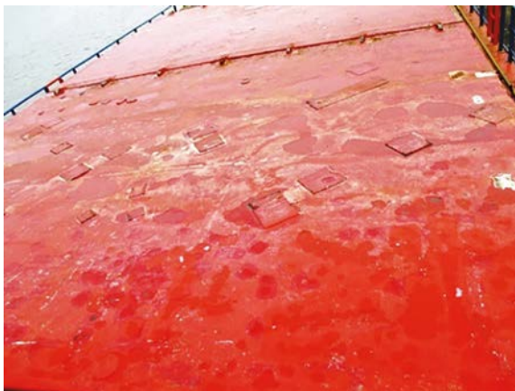
Figure 55.7: Multiple doubler plates on hatch top plating.
