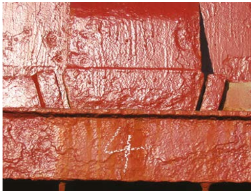
Figure 55.14: Excessive wear on the locator.
