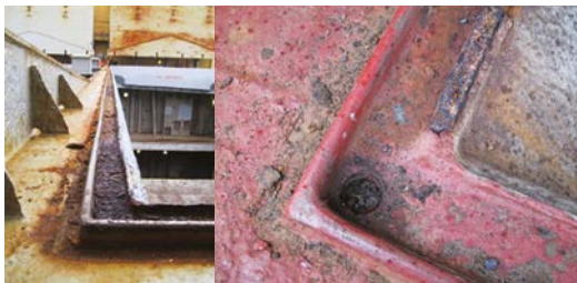
Figure 55.16: Blocked drainage systems.
