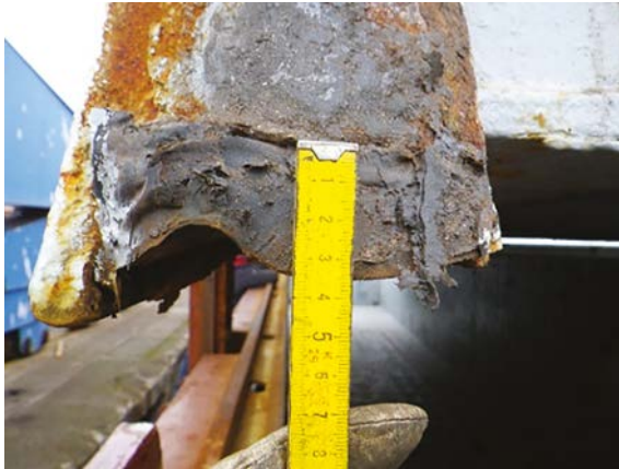
Figure 55.9: Permanent groove in packing rubber caused by overcompression.
