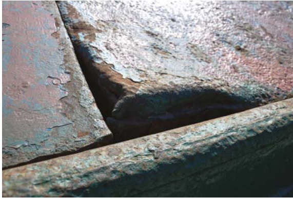
Figure 55.8: Damaged hatch cover which cannot be repaired at sea.
