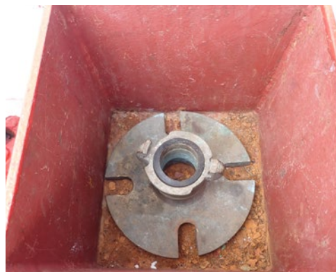
X International shore connection (ISC) connection not kept together with gasket bolts, nuts and washers.
