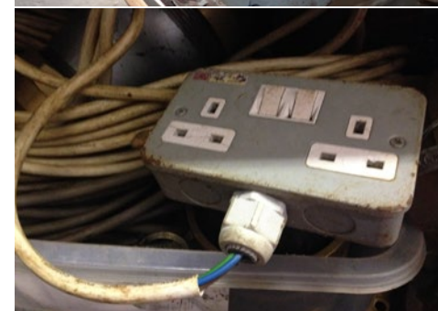
X Cable terminations should be secure. The cable jacket should be secured inside the termination – individual wires/conductors should not be exposed and junction boxes should not be taped in place.
