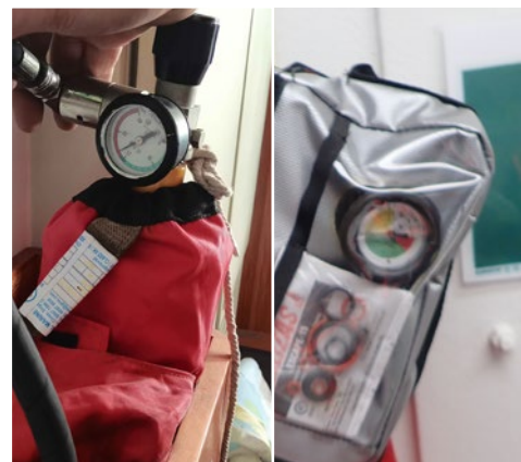
X EEBD gauge indicating an empty cylinder.
