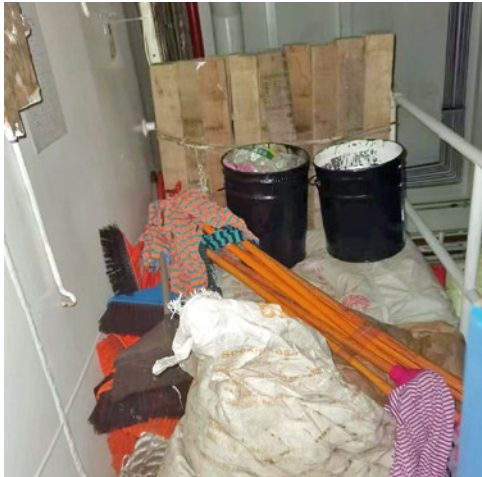
X Clutter making unsafe access to the vent flap.
