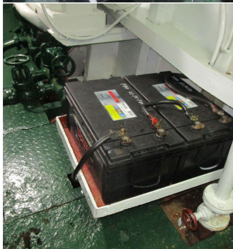
X Poor installation of batteries.
