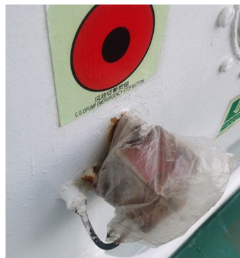
X Emergency stop not weather-tight.
