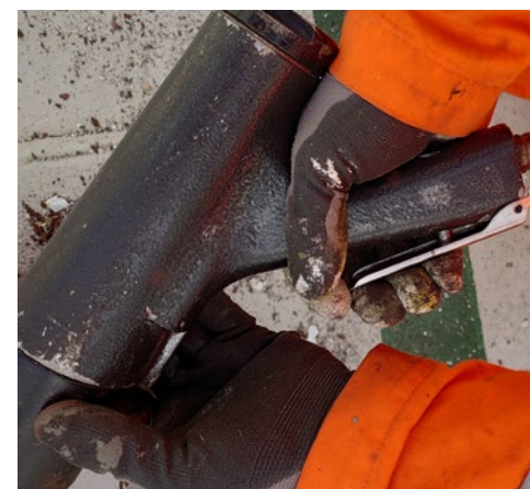
✓ Spring-loaded switch on the needle scaler is functional (not secured in ON position).
