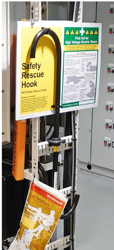
✓ Rescue equipment and first aid instructions posted in locations where there is a risk of electrocution.
