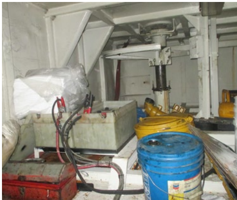
X Exposed batteries along with combustibles, chemicals and other disorganised equipment in steering gear compartment.
