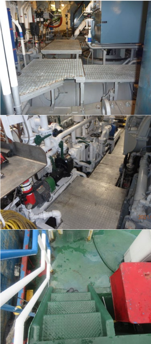
X Inadequate highlighting of changes in deck level
