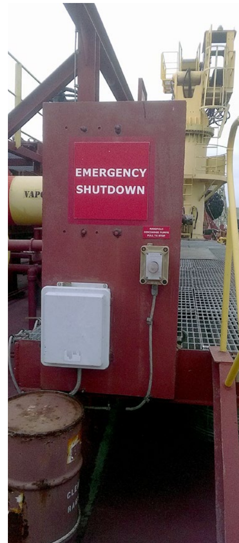
✓ Emergency shutdown and emergency stop buttons clearly signed.
