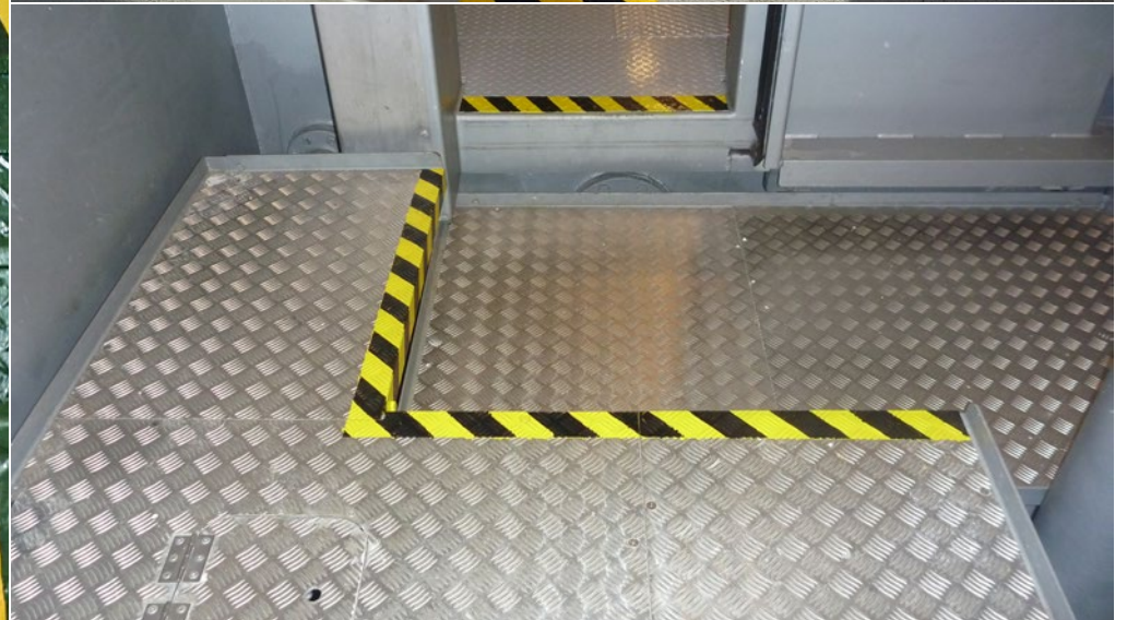
✓ Safe walkways and good highlighting of changes in deck level and permanent trip hazards
