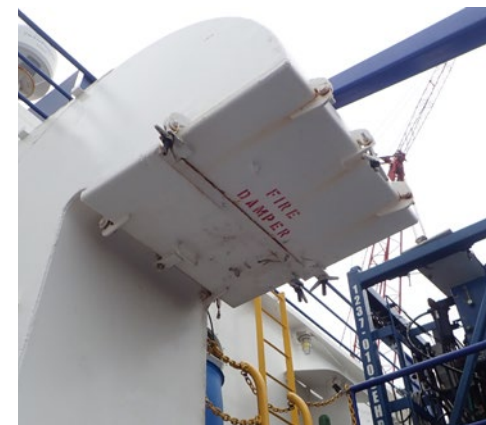
X Vent flap not marked to indicate the space/compartment served.
