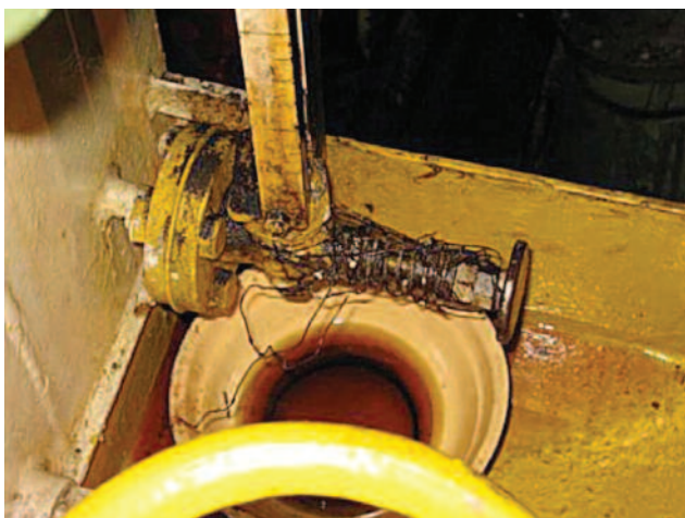
Self-closing gauge glass valve gagged with wire
