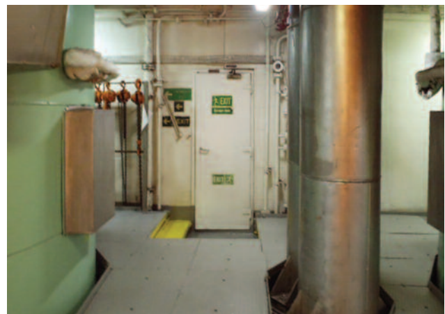
Poorly marked escape route and door
