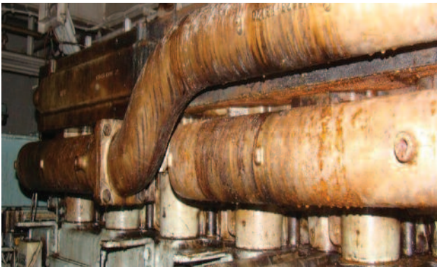
Exhausts completely uninsulated
