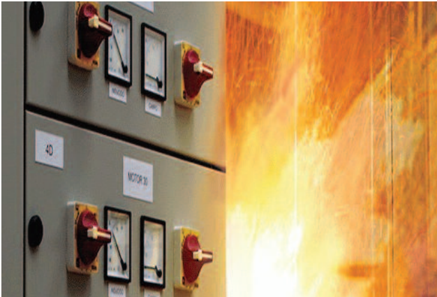
Arc flash incident
