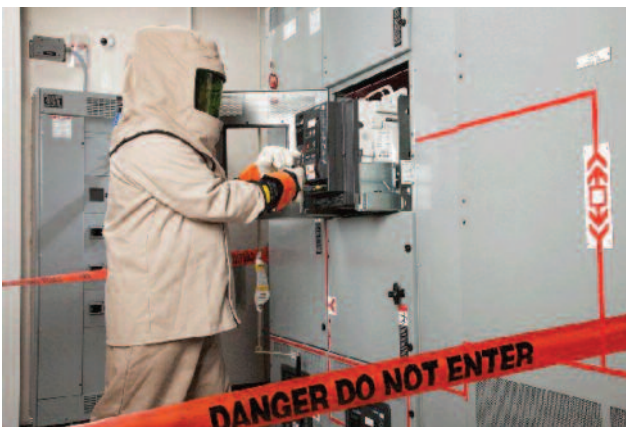
PPE to guard against the effects of arc flash
