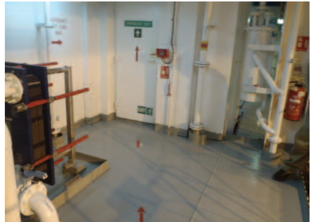
Well marked escape route arrows
