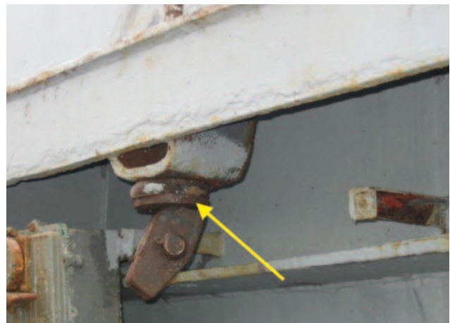
Overtightening of securing arrangements and crew member overtightening cleat with a spanner and cheater bar (top) until the rubber washer is reduced to pancake size (bottom)
