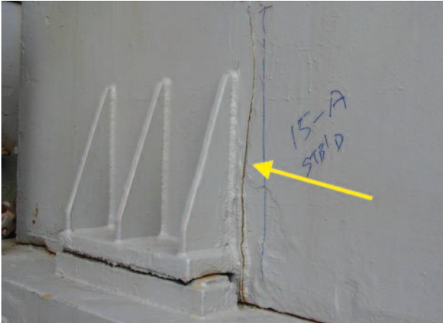
Improper repairs to bearing pad and a crack developing in the hatch panel side plating due to advanced bearing pad wear
