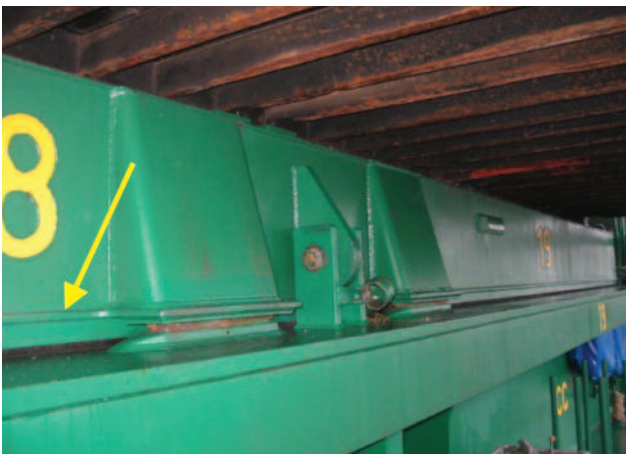
Operational clearance between the lower edge of the panel side plating and the coaming table
