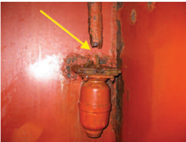
Corrosion wasted drainpipe
