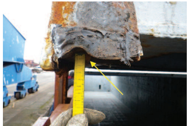
Deep permanent groove in packing rubber as a result of overcompression. Also note the off-centre permanent imprint
