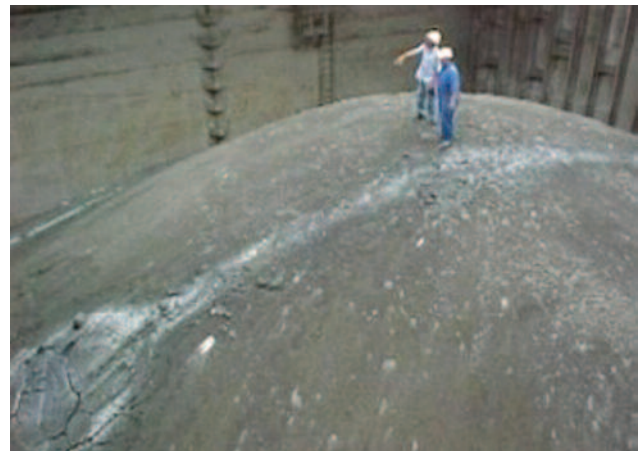
Evidence of leakage in way of the hatch cover cross joints
