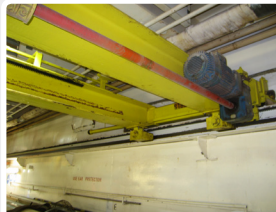
A typical engine room crane
